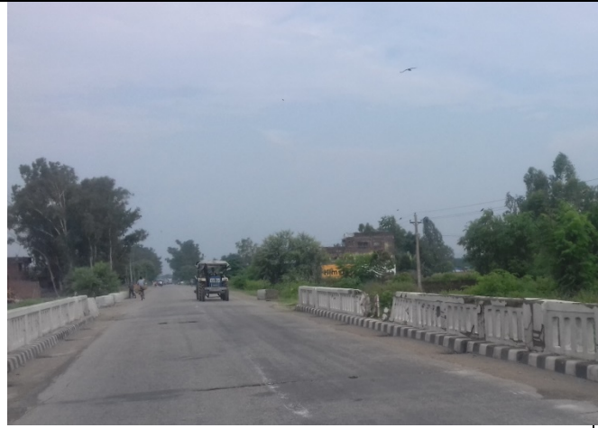
Bridge Railing broken on EW Highway, waiting for repair (Lahan-Mirchaiya)
