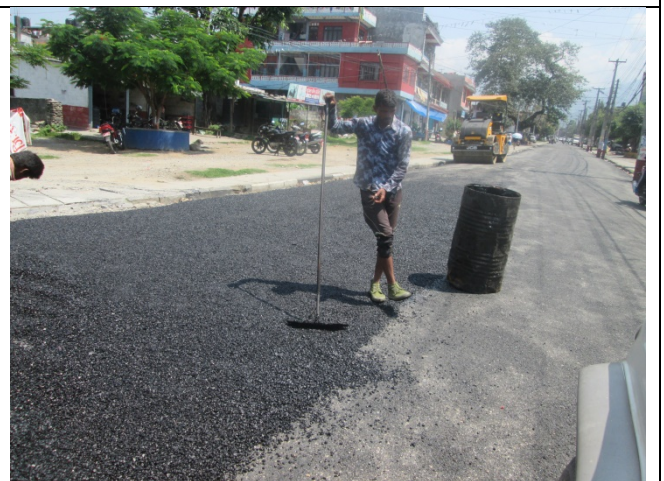
Patchwork on Pokhara city roads
