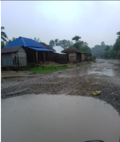
Large pot hole filled with water at Hanumannagar-Rajbiraj road
