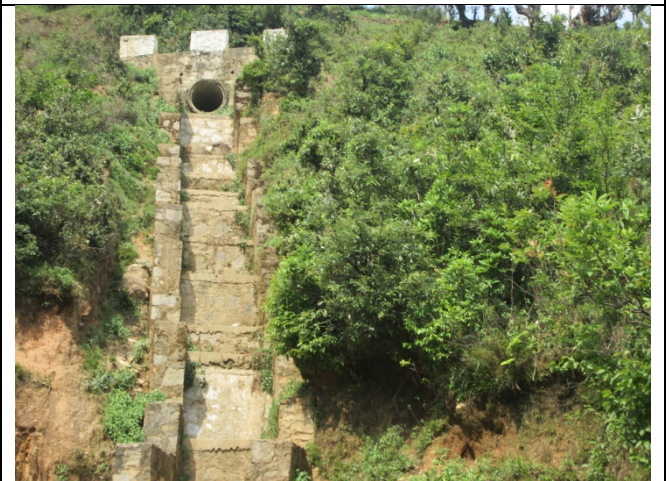
Cascading construction for safe disposing of cross drainage water, Attariya – Syaule road
