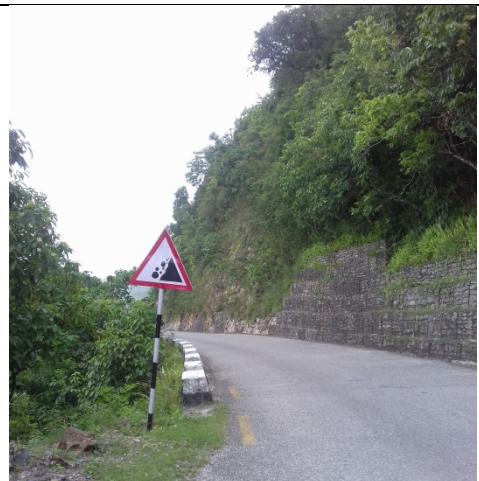
Road sign of landslide on Dhankuta-Bhedetar section
